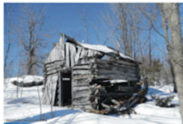
Abandoned building on the shores of Spectacle Lake, Elbow Lake Environmental Education Centre.
